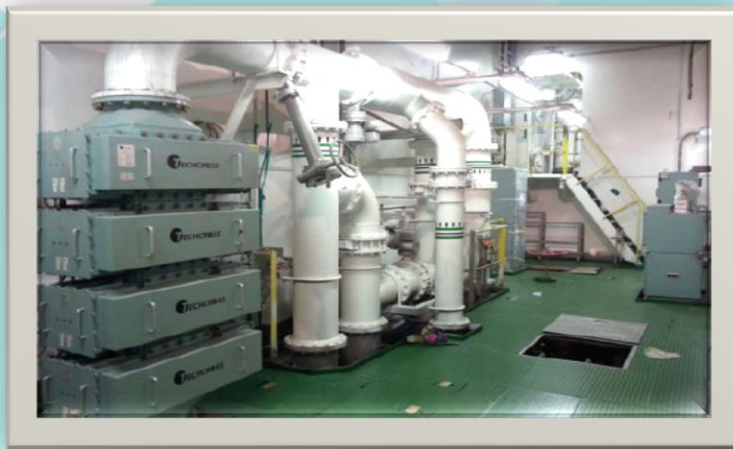
BWMS made by Techcross, Korea (Source: Techcross)
